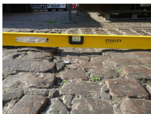
Photo 19: Zone 11 showing significant hazard and rounded/damage setts.
