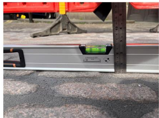
↑ Photo 04: Undulation of 3mm on walkway
