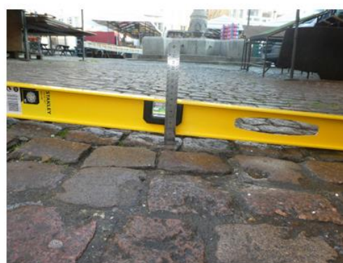
Photo 20: Undulation of 20mm on walkway in zone 3.
