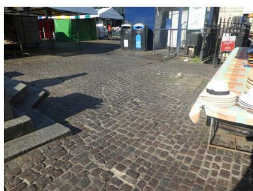
Photo 18: Zone 11 showing unevenness and worn pointing
