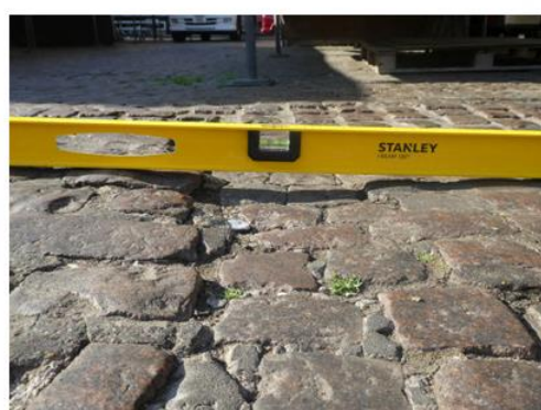
Photo 19: Zone 11 showing significant hazard and rounded/damage setts.
