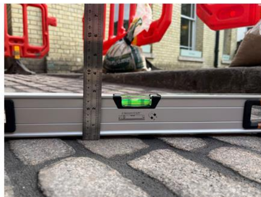
↑ Photo 02: Undulation of 6mm on walkway
