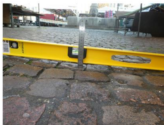
Photo 20: Undulation of 20mm on walkway in zone 3.
